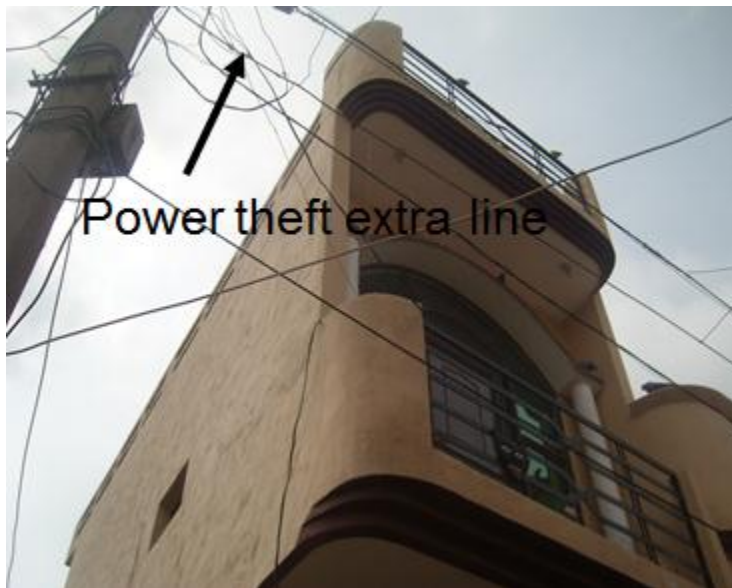
Figure 2. Shows the direct cut from one phase wire in residential area (Photo Credit: Deepa Madan).
