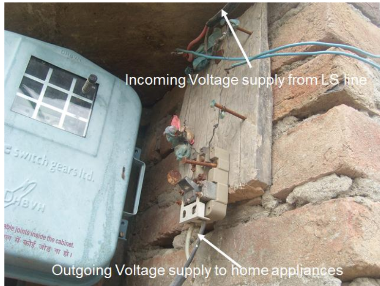
Figure 4. Shows bypassing the meter in residential area ( Photo Credit: Deepa Madan ).
